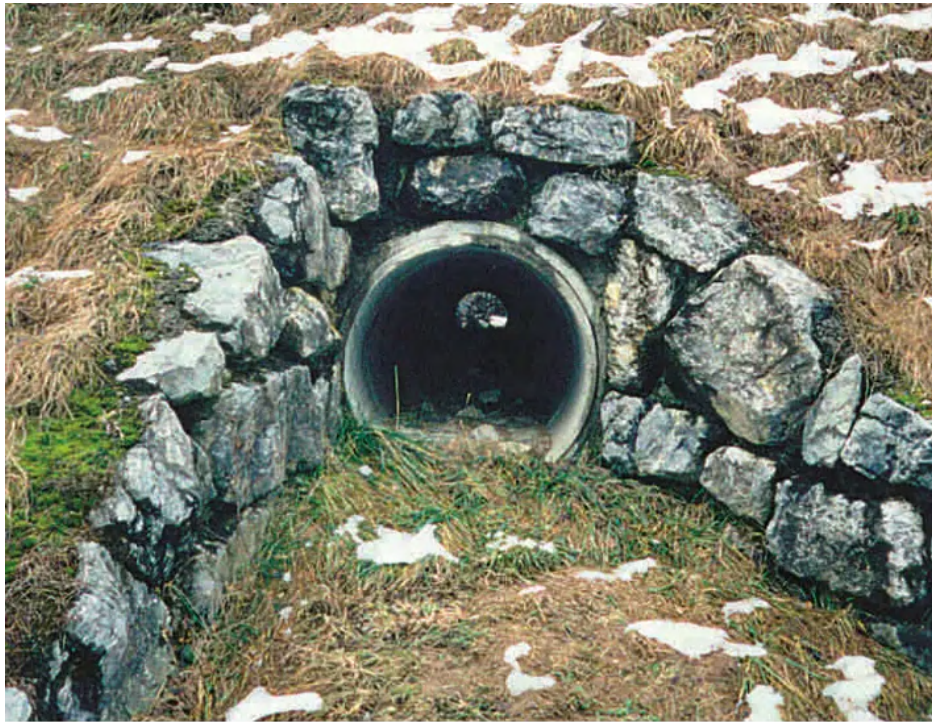
Figure 7.4.38 – Entrance to a small fauna underpass on the A8 in Switzerland (diameter 1 m). Stone walls, which in this mountain region are a common feature, guide animals to the passage. In such small structures maintenance tasks are difficult and could be often blocked by branches and other materials (Photo by: A. Righetti).
