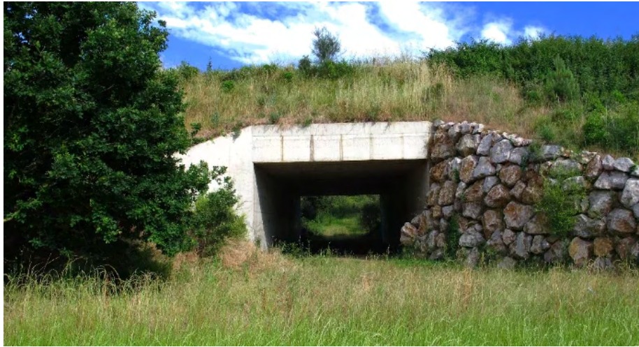
Figure 7.4.34 – Angled walls each side of the structure help to funnel animal movement to the entrance of the wildlife underpass under an irrigation channel (Photo by: Minuartia).
