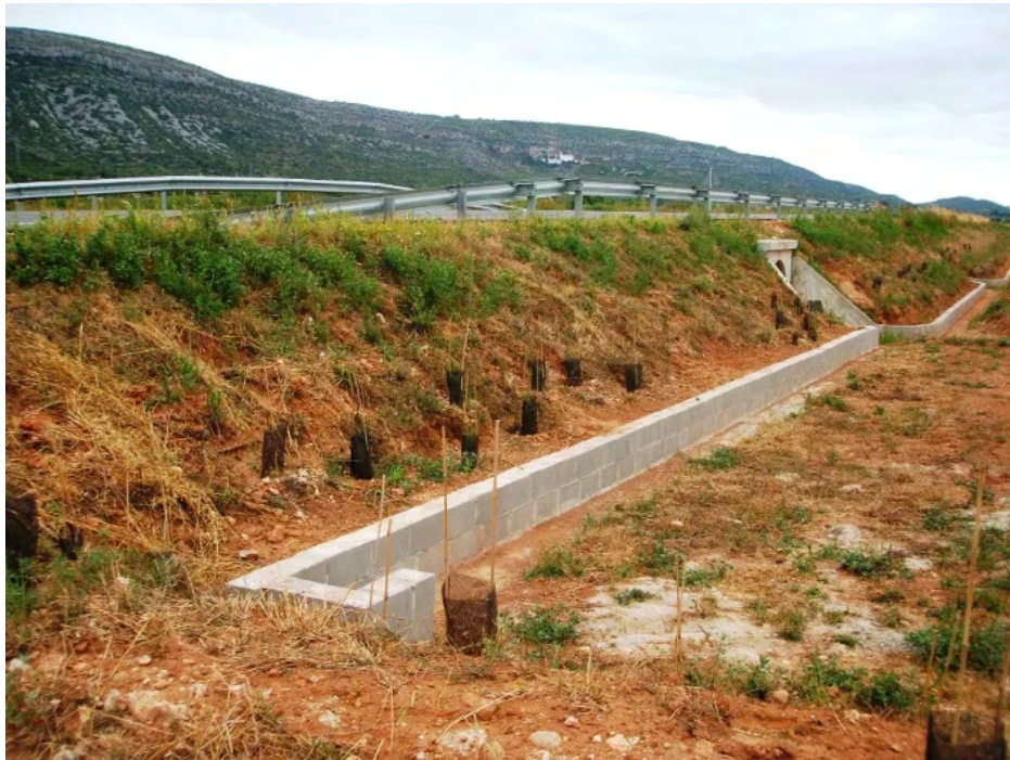
Figure 7.4.52 – The end of the amphibian passage guiding structure should be U-shaped to direct animals away from roads or railways and helps avoid access to the infrastructure (Photo by: Minuartia).
