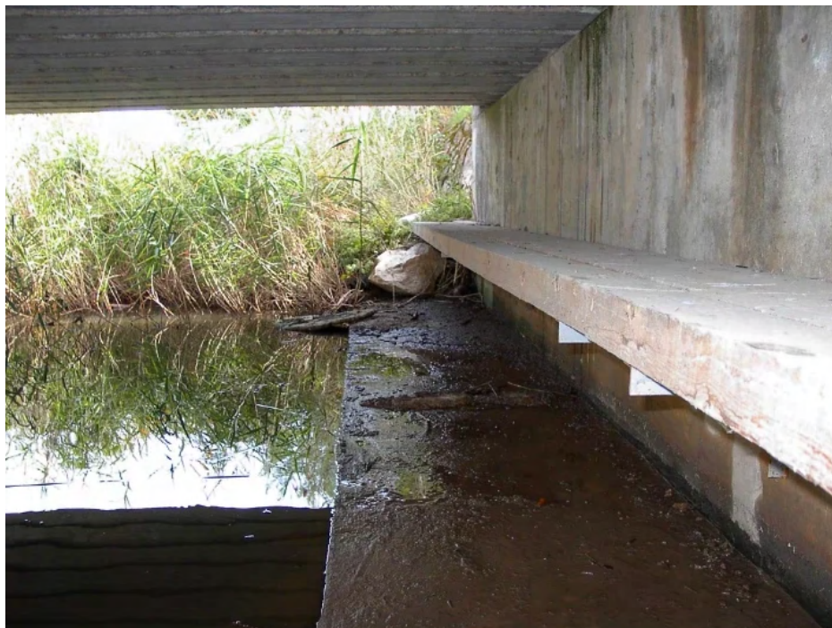
Figure 7.4.42 – Adapted culvert with two ledges to keep dry areas for fauna passage. The lower is part of the original concrete structure and the higher is a wooden ledge installed later to facilitate animal crossing when lower part is flooded. (Photo by: Minuartia).
