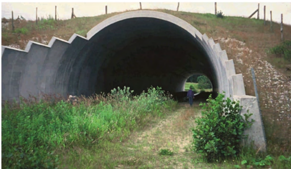
Figure 7.4.35 – Multiuse underpass in Denmark regularly used by wildlife (fox, badger, marten, stoat and polecat) as well as by humans and horses. The natural soil allows the growth of vegetation in some parts of the structure and reduces noise
