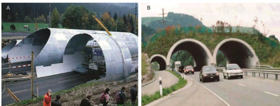
Figure 7.4.13 – A: Corrugated steel elements were used for this wildlife overpass in Switzerland (40 m wide), which was constructed across an existing road during widening. This allowed traffic to flow along one lane during the whole of the construction phase (Photo by: O. Holzgang); B: The same overpass after completion (Photo by: V. Hlavác).
