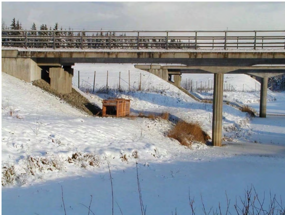
Figure 7.4.30 – Wildlife passages should be inspected periodically to avoid activities that can cause disturbance or damage to wildlife, such as this carnivore trap under a viaduct in Sweden. Photo by: J. O. Helldin.
