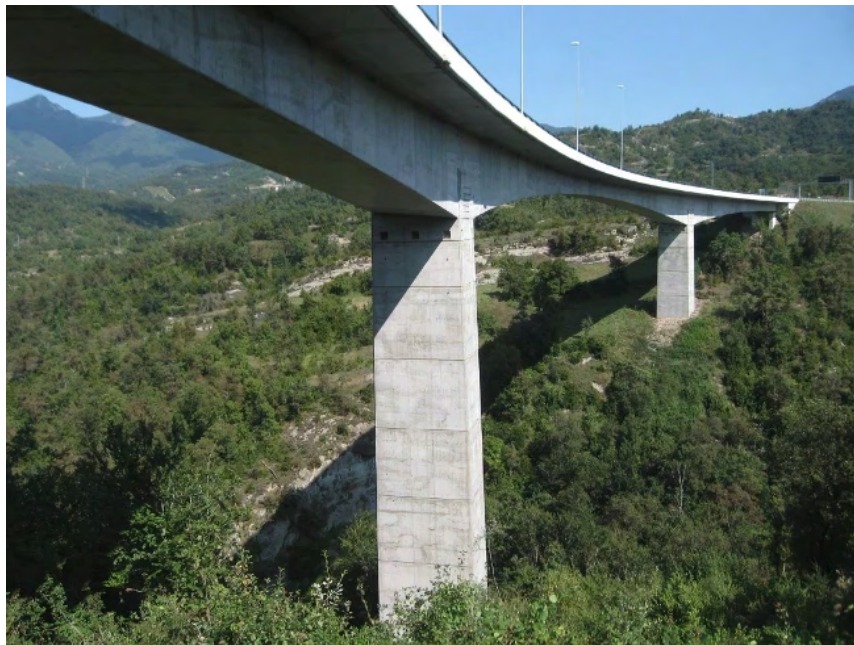
Figure 7.4.23 – Some construction methods, such as successive cantilever or pushed slab techniques, permit the building of viaducts while preserving the original vegetation and habitat conditions of the landscape beneath the structure, such as in this viaduct on the C37 in Catalonia, Spain (Photo by: Minuartia).
