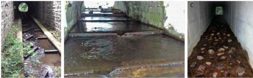
Figure 7.4.50 – Solutions to adapt existing drainage structures to enhance opportunities for fish passage – not recommended for any new infrastructure where best options are wider structures which allow the restoration of the stream and natural embankments at each site. A: Installing weirs stabilises the reconstituted substrate but also concentrates low flows and provides resting areas for fish. Lateral dry passages also allow terrestrial mammals to use this passage (Source: Cerema, 2021); B: Installation of weirs in a passage that is only suitable for fish (Source: Cerema, 2021); C: Stones fixed into the substrate achieve the same objective as weirs but are not suitable for mammal crossing (Source: S etra, 2013).
